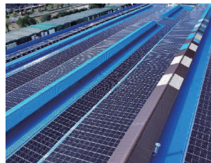
AIKO's PV power station project supports Taishan Gypsum's energy transition
