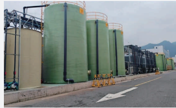
Workshop wastewater classification and recycling device
