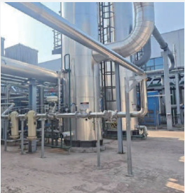
Yiwu Base Air Compression Waste Heat Recycled System
