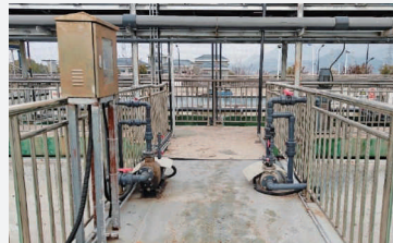
Wastewater Recycling and Reuse System
