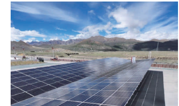
AIKO's N-type ABC dual-glass 645W modules power the world's highest-altitude integrated PV-storage supercharging station
